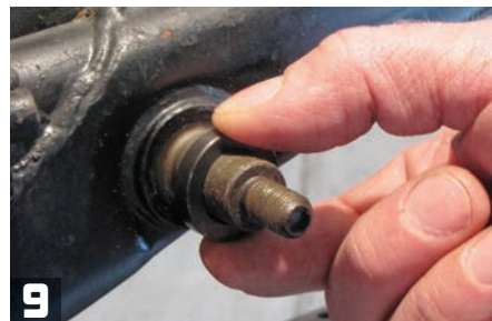
Supplied spacers were needed for this install when hanging the new shocks.
